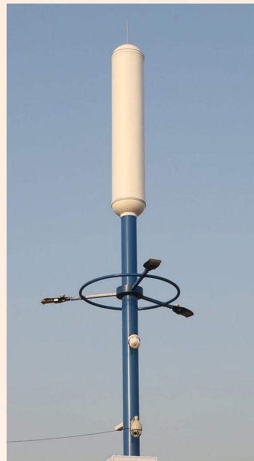
Image 28: A multi-utility "Smart Pole" installed in Visakhapatnam Smart City. A network of these poles have facilitated wi-fi connectivity in public areas across different cities. The mission has helped expand access to the internet in the selected cities. Source: Visakhapatnam Smart City
