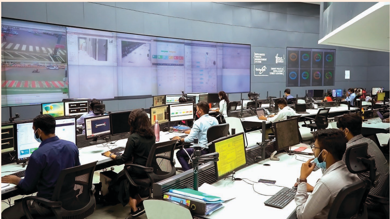
Image 27: The 100 SCM cities have operationalised ICCC as the central hub for urban management. These state-of-the-art centres utilize the latest technologies and enable seamless coordination across various sectors. Source: Bhopal Smart City.
