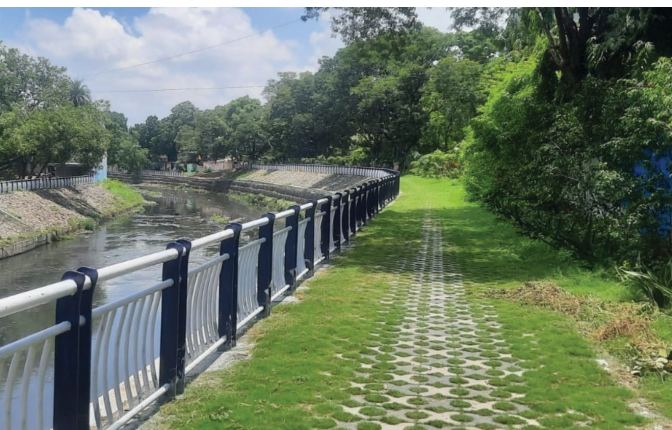
Image 17: Indore Smart City constructed retaining walls alongside a pilot stretch of Saraswati river to ensure unobstructed flow of the river and implemented measures to prevent sewage and untreated water from entering the river through smaller drains and nalahs. The riverfront development has added 0.4 sqkm of green space to the city. Source: Indore Smart City.
