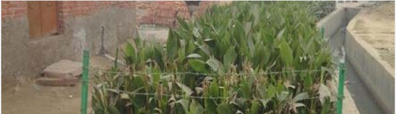
Image 3.6: Planted filter bed for root zone treatment of wastewater
